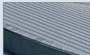
Metal cladding: Example of zinc metal cladding to roof and elevational returns
