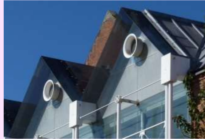
Crisp, high quality contemporary roof detailing, particularly stemming from the fine glazing detail.
