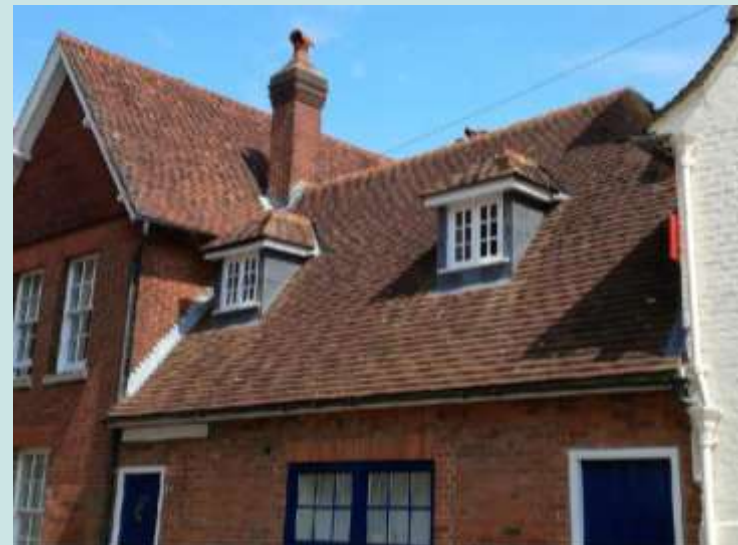
These dormers utilise excellent materials and detailing, and the scale and proportions relate successfully to the existing roof.
