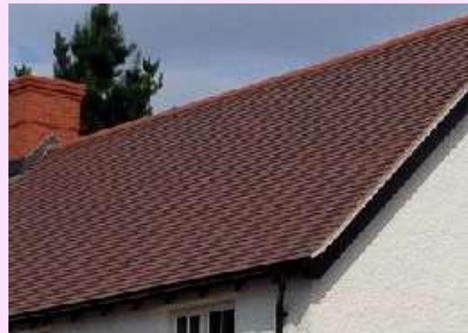
Successful traditional eaves detailing, note the benefits of the dark, open eaves.
