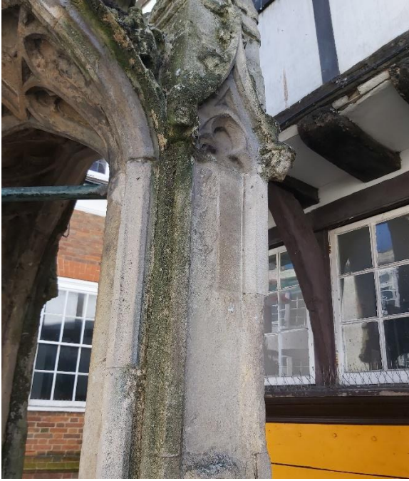
Fig 22 – runoff from guano deposits causing staining to the stage 1 shafts
