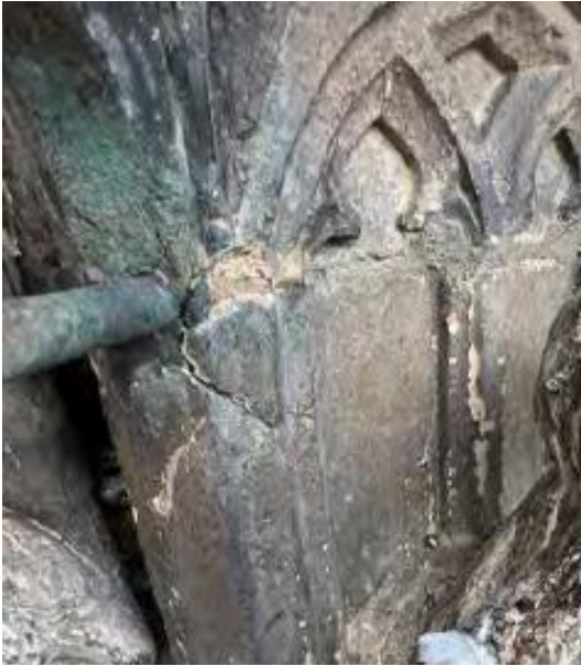
Fig 21 – tie rod junction to masonry with spalling masonry at junction.
