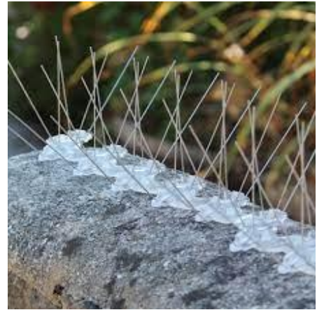
Fig 31 – spikes attached to the top of a wall.
