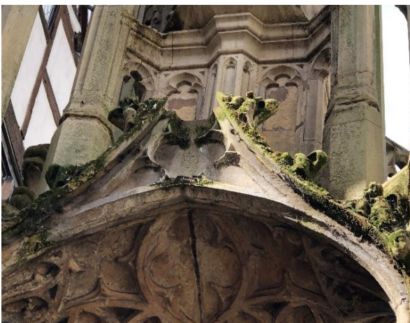
Fig 14 - view of the east facing gable arch where the finial has been lost.
