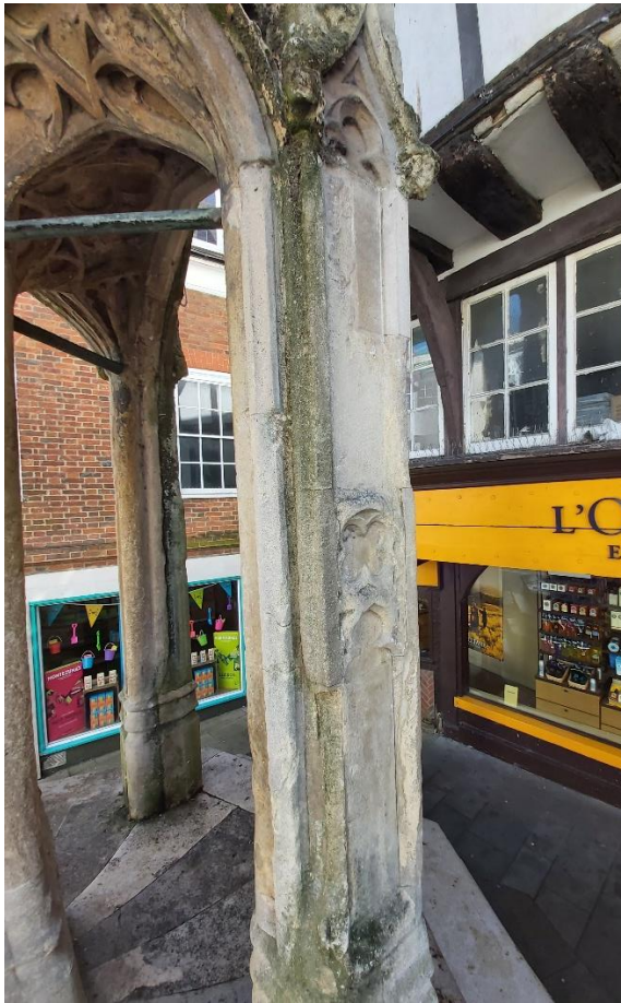
Fig 13 – the outer shafts at stage 1 have been the subject of continual repair and replacement stone could be considered where a previous repair has failed. However, where the moulding has been lost or damaged and not yet repaired we would be hesitant to propose replacement because of the potential loss of original fabric that would be required to put in place a robust repair.
