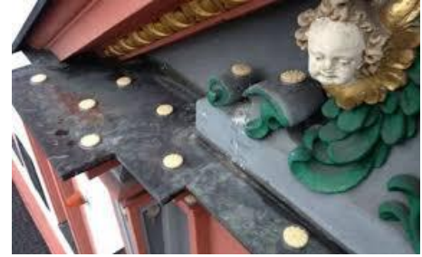
Fig 33 – Optical gel trays fixed on top of a cornice.
