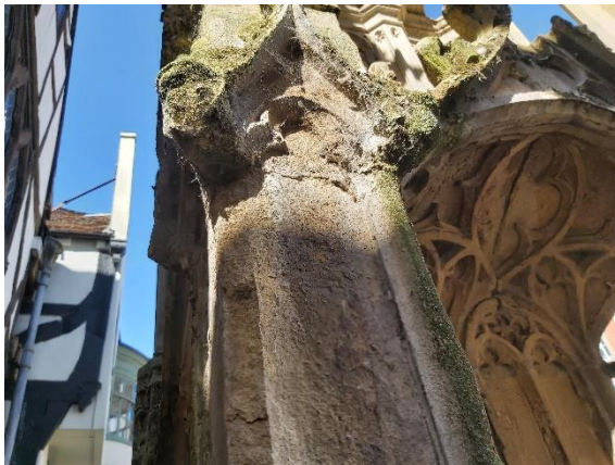
Fig 12 – friable masonry around the outer shafts at stage 1.
