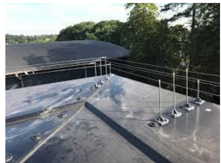
Fig 29 – bird wires with supporting posts.
