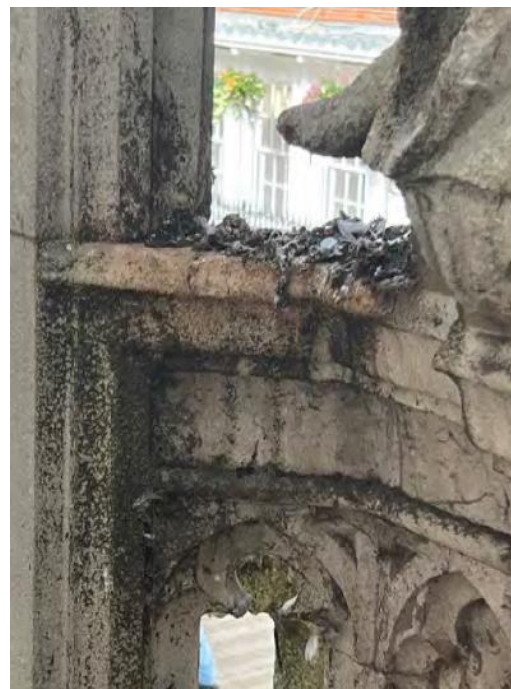
Fig 24 – Stage 2 area around the feet of St John the Baptist on the south elevation.
