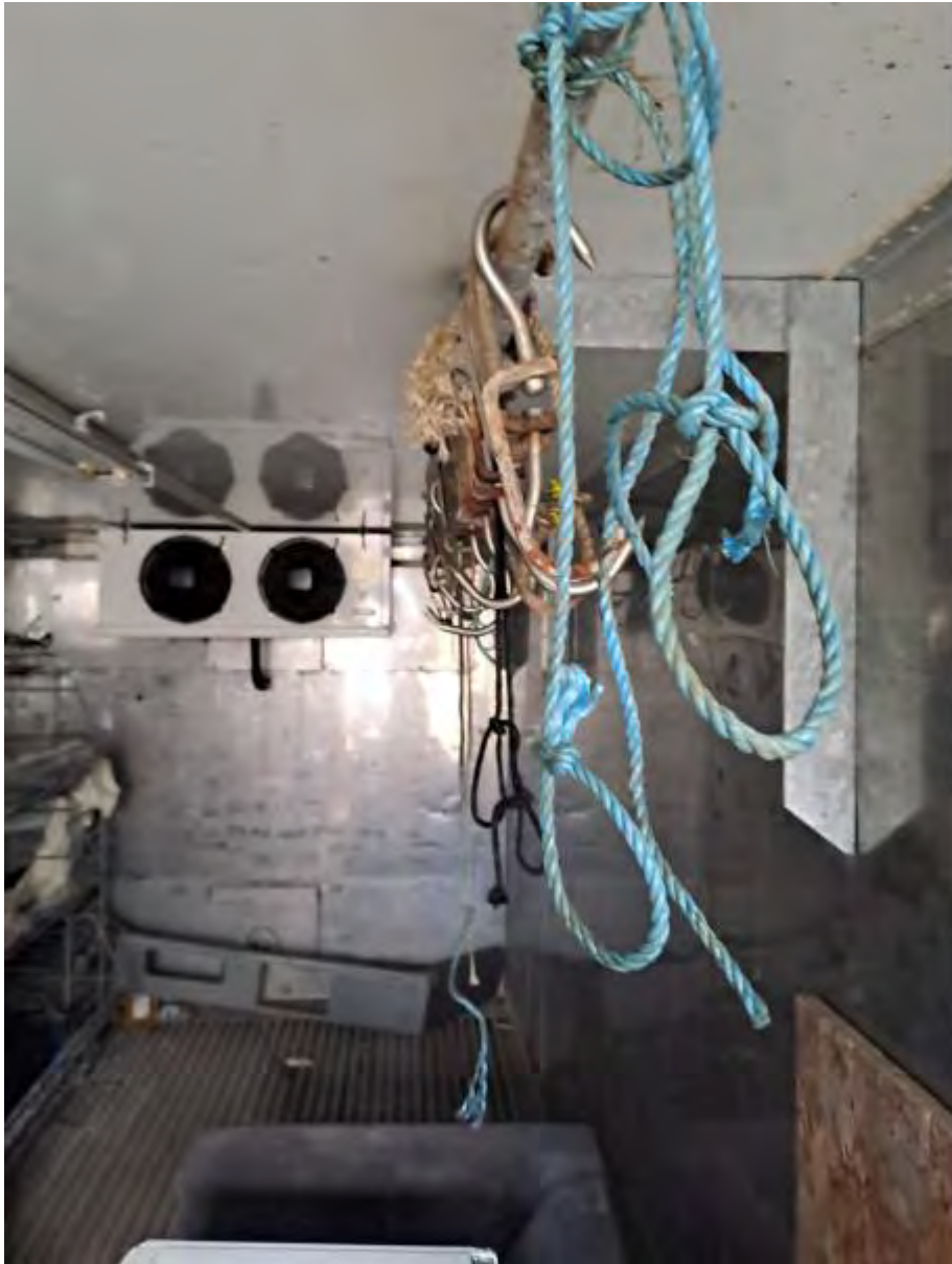
Interior of butcher's freezer unit
