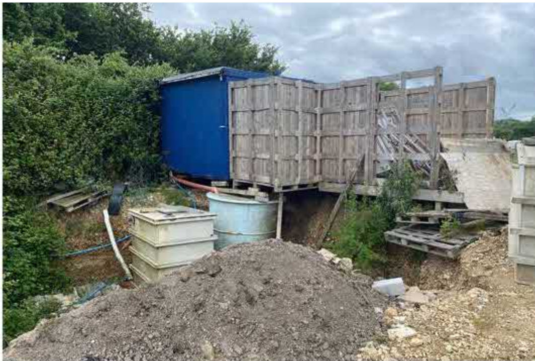
Figure 1 Septic tank and installations
