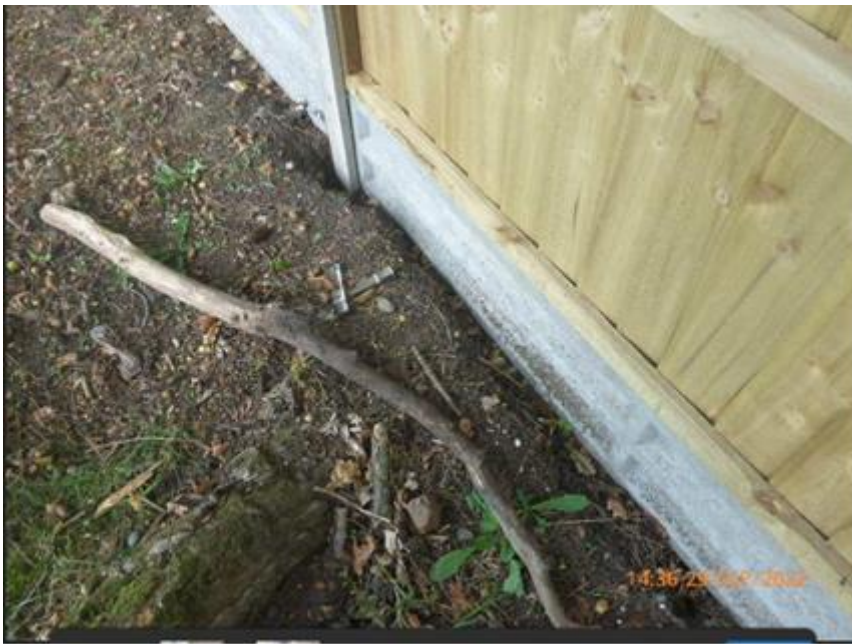
The above photo shows how close the development is to a major structural root, let alone all the feeder roots which were damaged as a result of the excavations.
