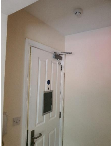
3. Room 6 door not effectively self closing
