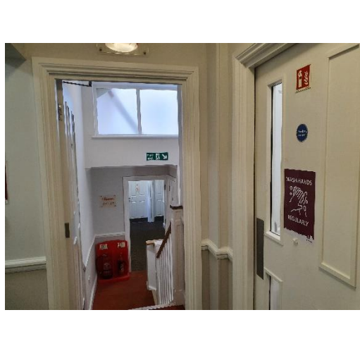
4. Door to 1st floor dining room lobby not self closing
