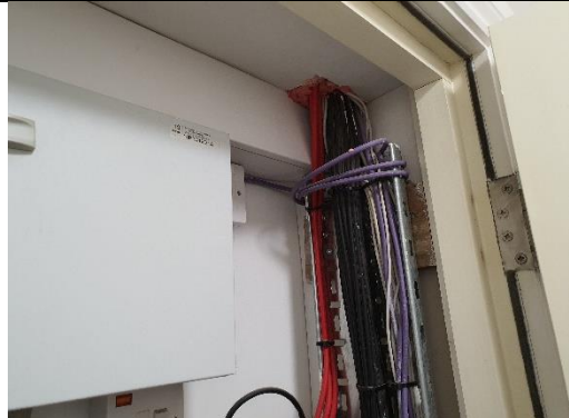
6. 1st floor electrical cupboard fire stopping inadequate
