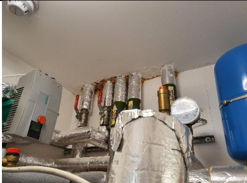
5. Boiler room fire stopping inadequate
