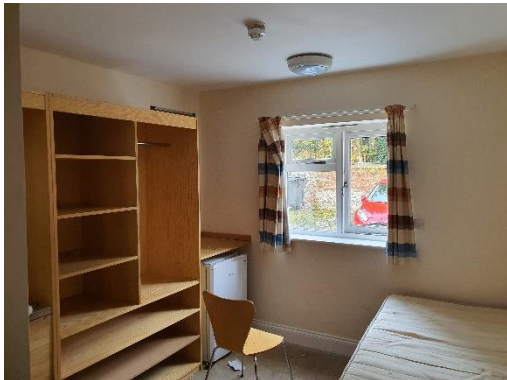
1. Room 6 smoke detection
