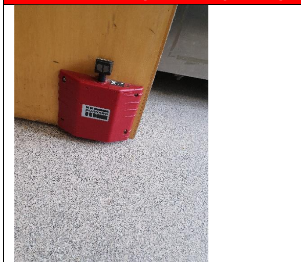
12. Acoustic hold open device (disused)
