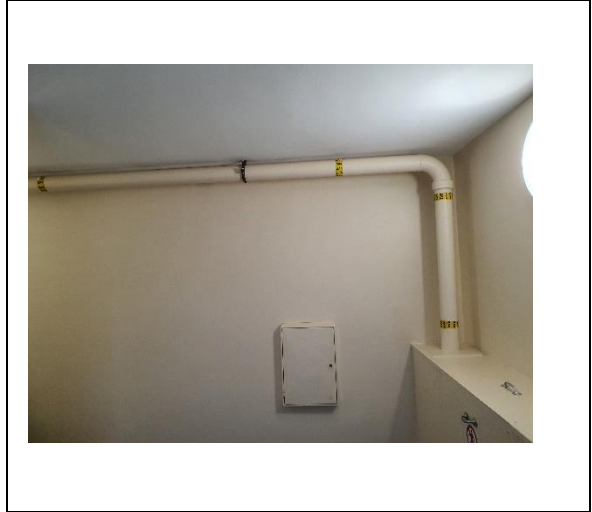
2. Gas main pipe
