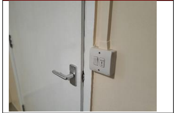
6. Zone 3 laundry – door not fully closing
