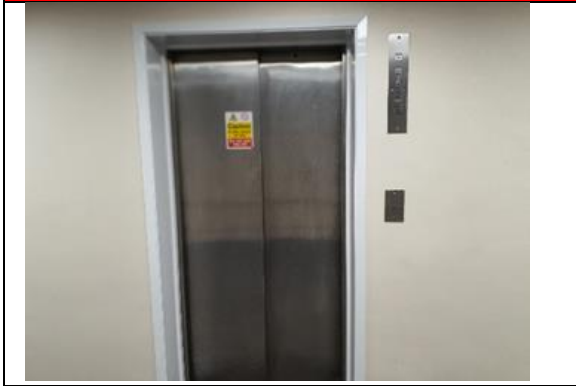
5. Sign on lift – do not use in fire
