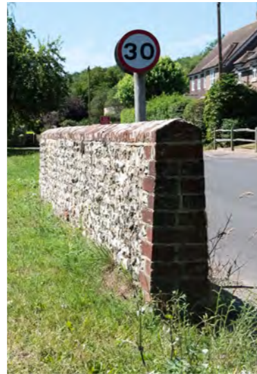
Left: Flint and brick wall Old Barn Crescent – good repair showing tapering profile of flint wall
