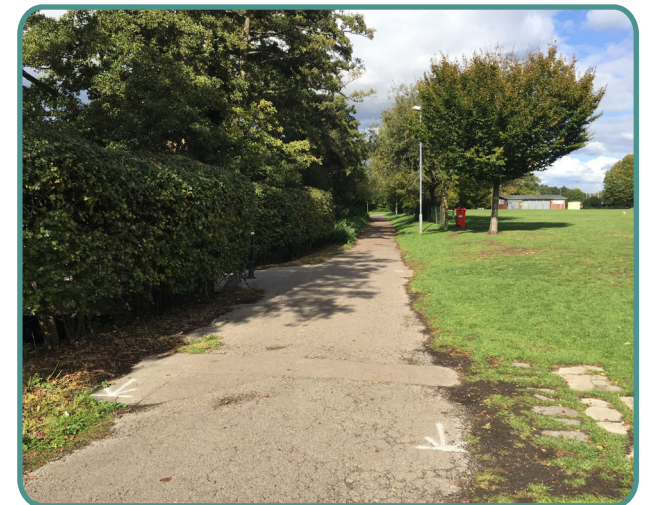
Existing path in need of upgrading
