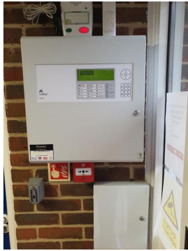
1. Main fire alarm panel
