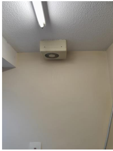
7. G/f Laundry vent into ceiling area
