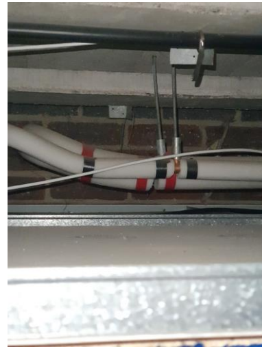
2. Services above false ceiling
