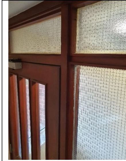
6. 4 th floor stair door -10mm gaps and 10mm overhang
