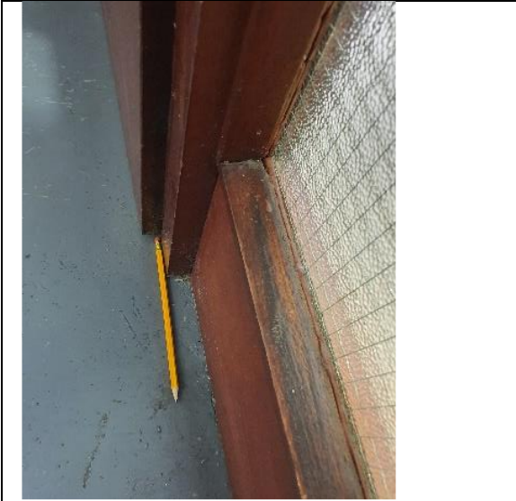
3. 6 th floor stair door warped (>18mm)
