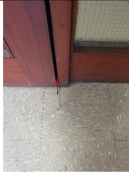
4. 6 th floor corridor door – 10mm gaps
