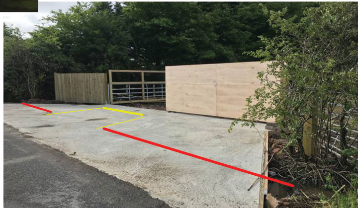
New gates installed yellow lines - old gate entrance overlaid on view red lines - removed hedge row
