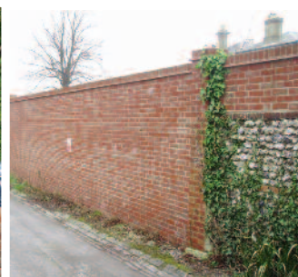
A new severe blank wall
