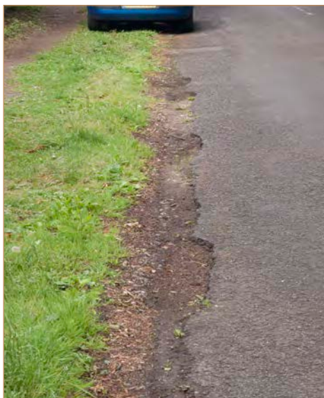
Damaged road edge
