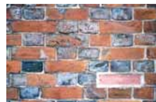
Wrong Mortar used in repair
