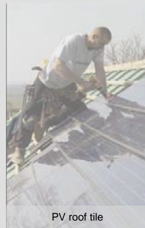
Roof mounted PV array
