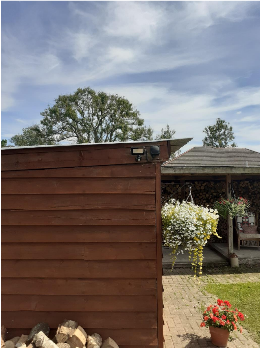
Security light on Northern corner of original building. Note that this light is directed in the opposite direction of No.6 and approx. 7m from their boundary.
