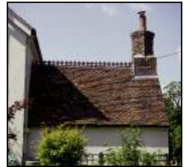
Riversdale - Interesting patterned tiling, for the Headmaster's house. Also on Jays Croft - the former school.
