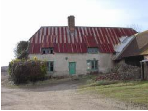
This derelict building had consent for renovation/conversion. The countryside benefits from such buildings brought back into use.
