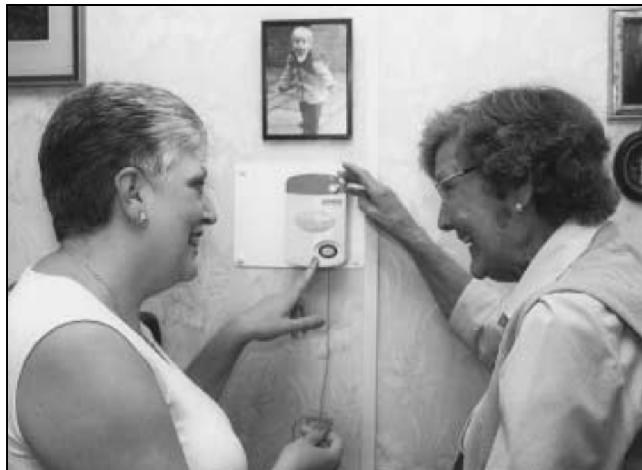
Community Alarm Service Manager, Lynn Curtis, with the newly installed Warden Call System in the home of Mrs. Pat Richardson at Airlie Corner.
